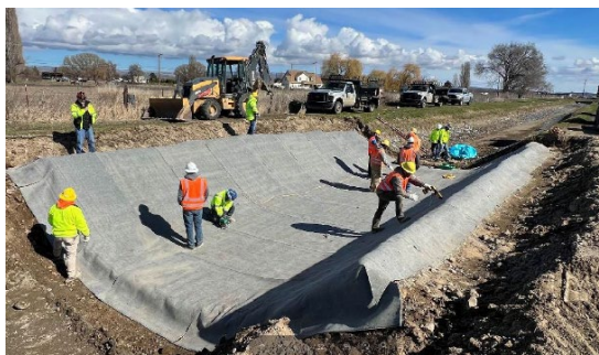
Field demonstration of concrete cloth installation to reduce seepage in a canal.
